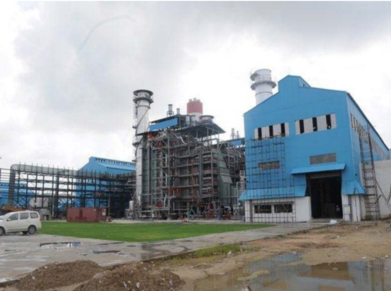
Bathinda combined-cycle power plant, Punjab, India
